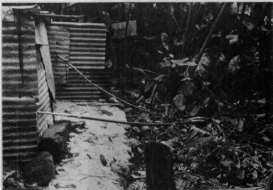
Figure 4. Pipe leaving pump enclosure and entering taro patch near Epinup Village.
